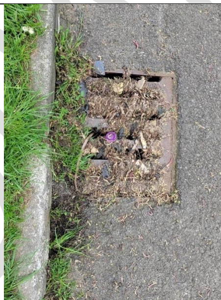
Figure 9: "Blinded" Gully on Blind Lane
