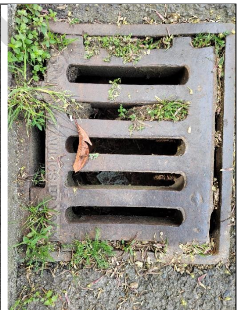
Figure 10: Gully on Blind Lane
